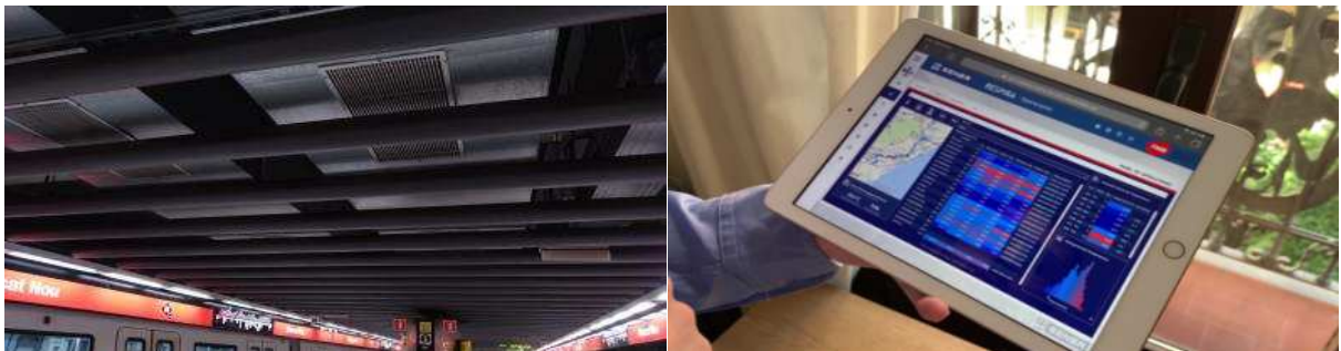
Ventilation of a station on line 1 of the Barcelona metro and system monitoring console / © SENER
